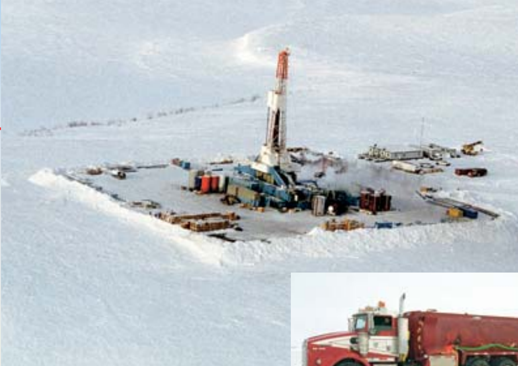
Northwind Industries helped build a pad for this new rig and gas well site operated by the Mackenzie Delta Partnership. The pad is located 117 kilometres northwest of Inuvik on Ellice Island.
