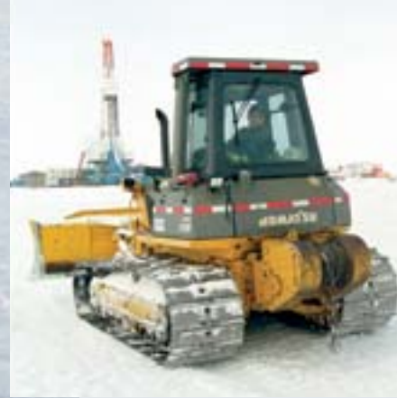
A Northwind Industries operator uses a Komatsu D41P dozer to level snow and ice while crews help construct a flare-unit site for testing near the gas well location at Ellice Island.
